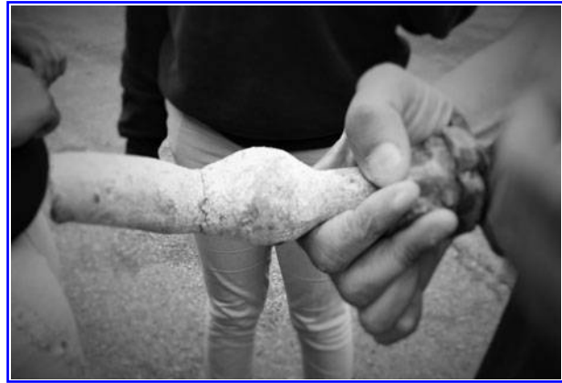
FIG. 1. Part of a lead service line removed from a New Orleans home, Faubourg Tremé (May 2, 2016). Credit: Adrienne Katner.
